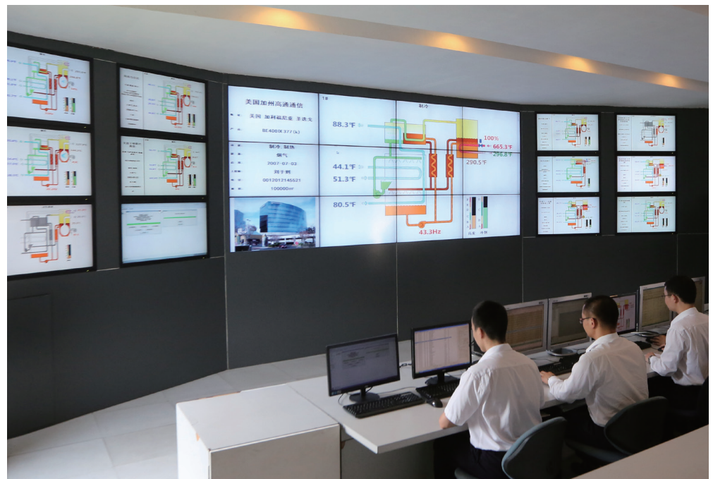
Global Internet Monitoring Center for BROAD central air conditioning. It has been operating since 1996, known as the pioneer of "internet +".
